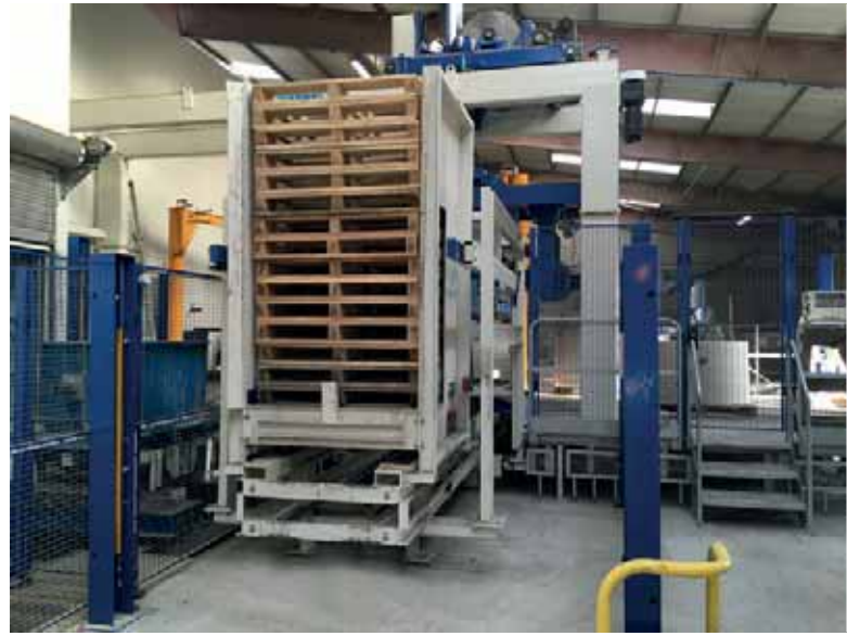
The production line is fed with pallets via a pallet storage system that keeps more than 20 pallets.
