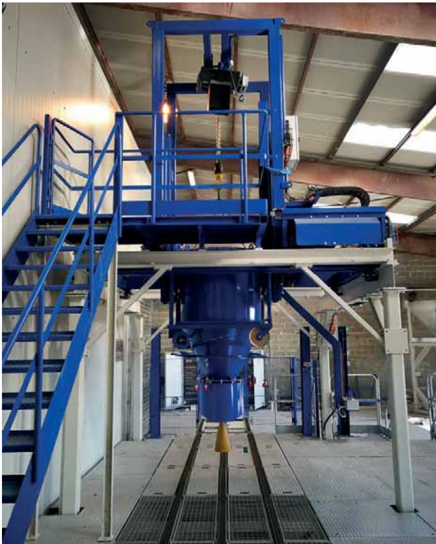
Molds filling system
