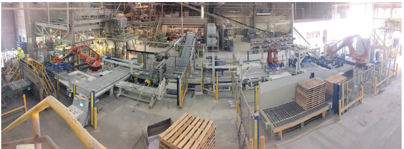
Complete new cubing line with three robots, conveyor system and splitter
